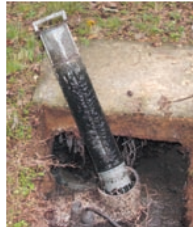
System inspections are a key component of management programs. Clogged septic tank effluent filters (above) can trigger calls for needed service, but regular inspections tailored to system type, setting, and use profile provide a better approach for ensuring long-term system performance.
