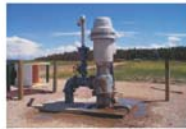
Water supply well in rural Wyoming.
