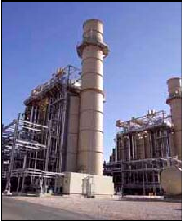
Silverhawk Generating Station
