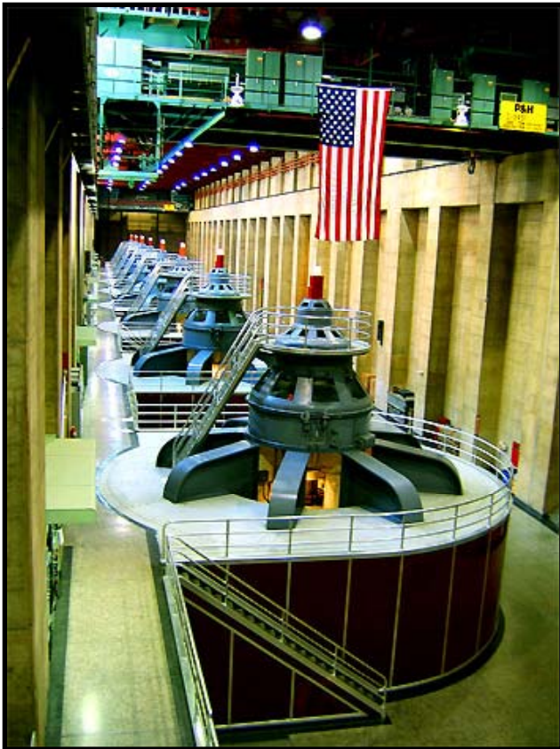
Hoover Dam's turbine room
