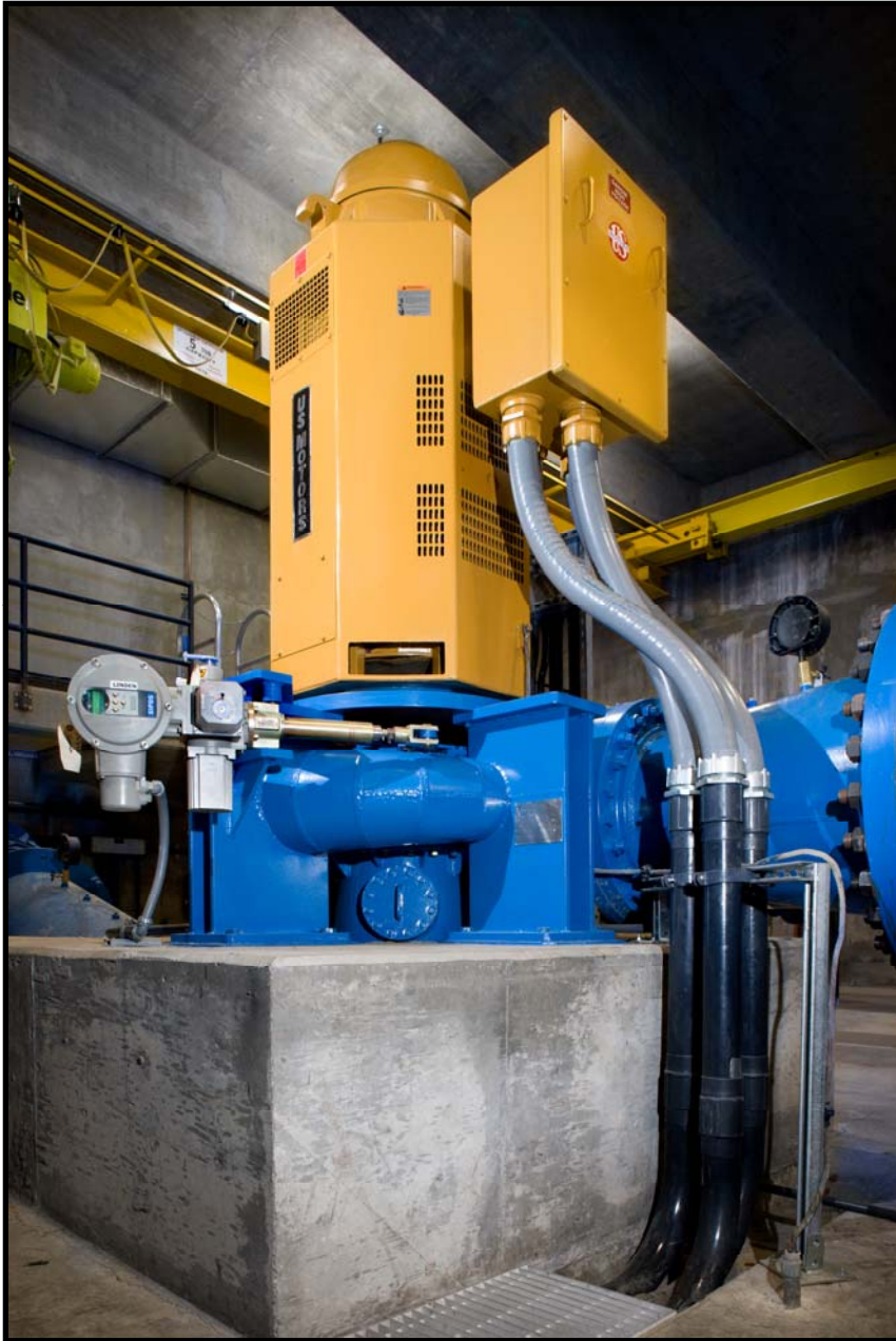
SNWA Member Agency pumping station
