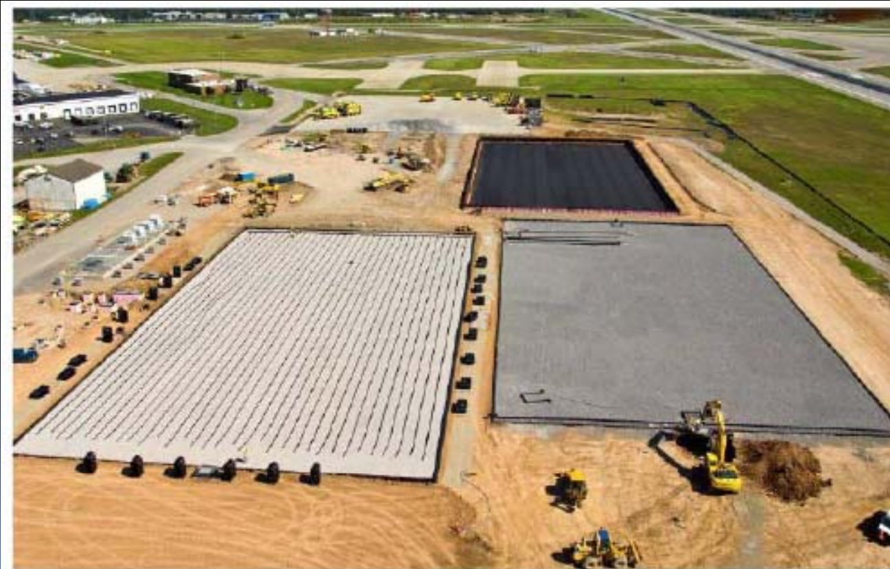
Figure 1. Vertical subsurface flow (VSSF) engineered wetland under construction at Buffalo, New York.
