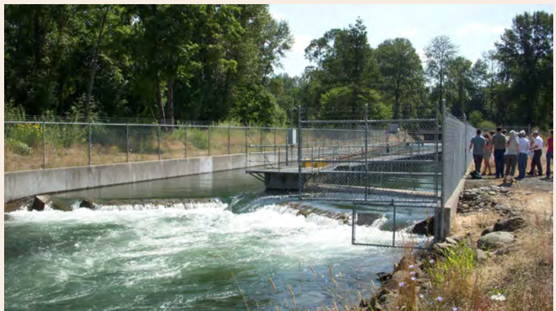
Santiam Water Control District fish passage structure near Turner, Oregon; expensive upgrades to comply with current Willamette Basin Biological Opinion requirements will impact industry in the basin.
