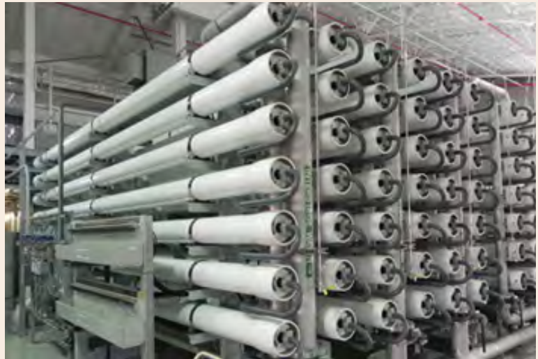
El Paso, Texas is the site of the world's largest inland desalination plant. This plant represents a forward-looking strategy in water supply—not only for a region but also for a world that is increasingly challenged by short supplies of fresh water.
