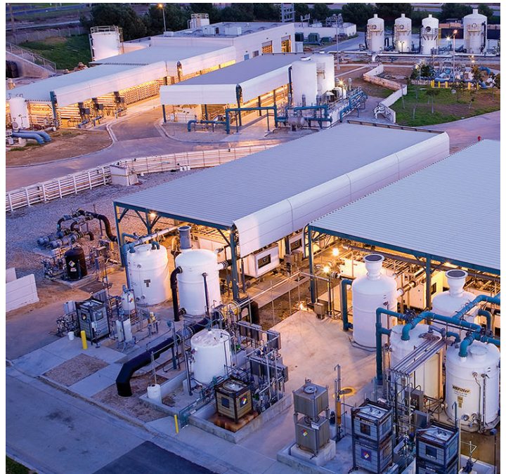
West Basin Municipal Water District's Edward C. Little Water Recycling Facility in El Segundo, California, produces and delivers five different types of customer-specific recycled waters.
