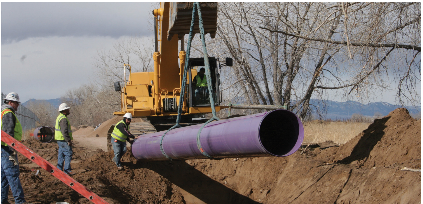
Denver Water contractors install a purple pipe used to deliver recycled water in northeast Denver, Colorado.
