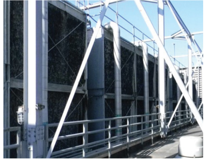
GlaxoSmithKline (Upper Providence, Pennsylvania) air handler condensate is reused by their cooling towers, resulting in 9 million gallons water savings in 2019, equivalent to $140,000 in cost savings and a 14.3 percent reduction in water use.
