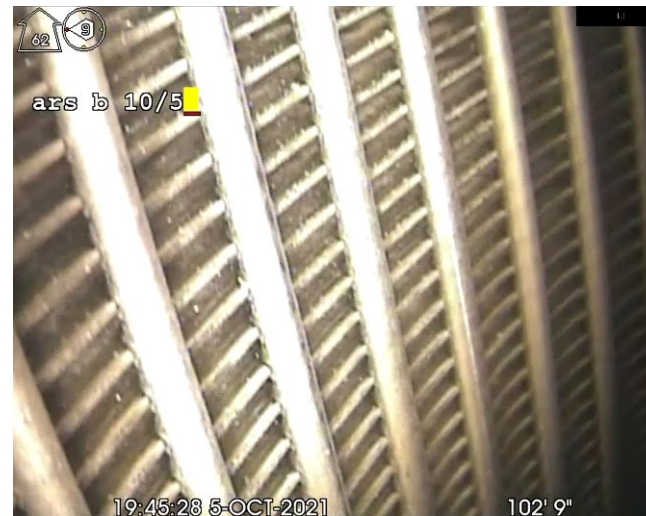
Injection Well B after rehab
