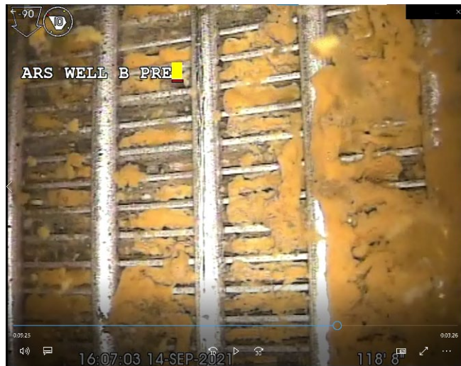
Injection Well B before rehab
