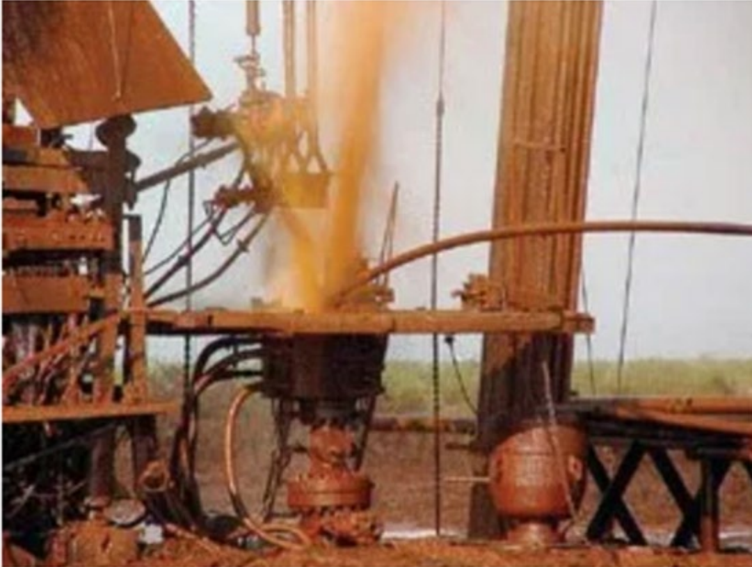
Blowout during workover to clean out fill in miscible CO2 injector
